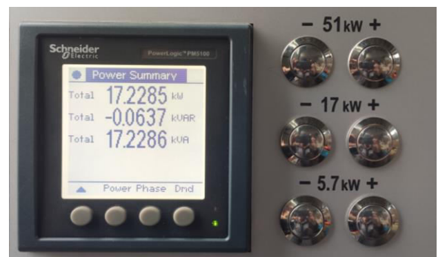
Figure 6. Control panel with power meter PM5110 series.
