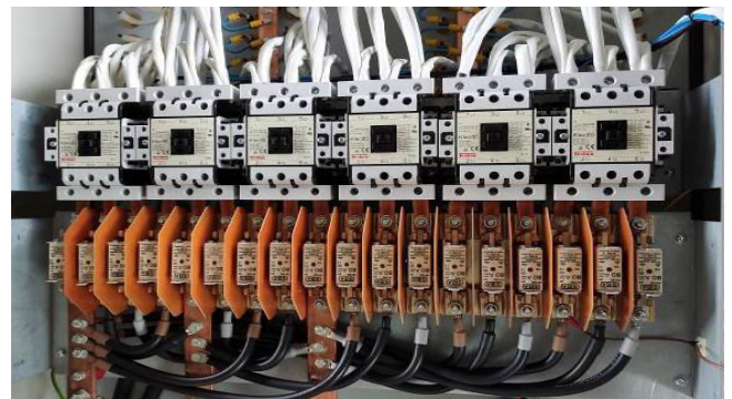
Figure 4. Main 6 contactors with connected set of heating elements
